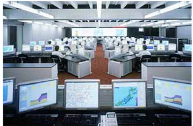
Fig. 6 : DC powered monitoring and management system: MaRIA.
